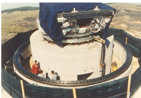
Figure 3 – the rotation system of the TNG while being installed on the external cylinder of the pillar.
